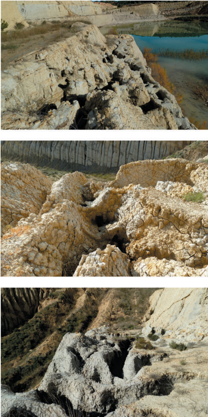
Figure 2. Tunnel erosion, piping, at benches of highwall terraces, at the Pastor I quarry.
