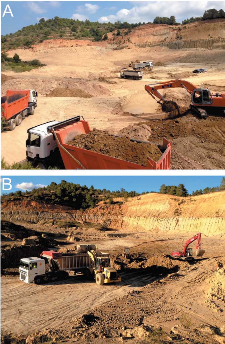
Figure 4. Photos of June 2015 showing the simultaneous process of exploitation and restoration at the Aurora quarry. (a) The two tipper trucks and the excavators, in foreground, are handling topsoil for restoration; the two box trucks and the loader the centre of the image are loading and transporting clay for the cement plant. (b) The loader is loading clay at a box truck (exploitation) whereas the excavator and a bulldozer, to their right, are regrading the final surface according to the geomorphic restoration plan.
