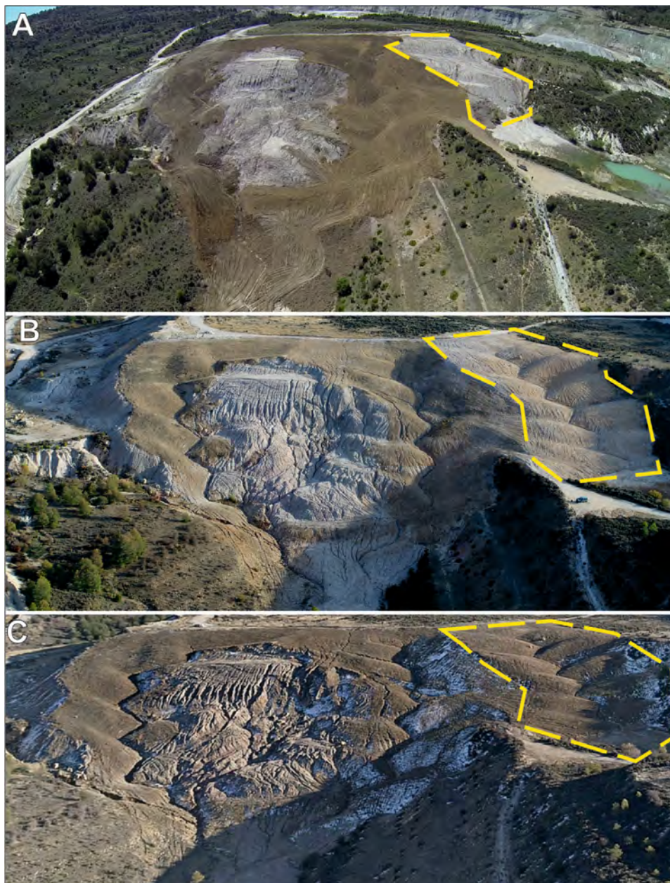
Fig. 8. Oblique aerial views of the geomorphic stabilization undertaken in the Nuria landslide: at the end of the construction, in May 2015 (A), in November 2017 (B), and in February 2019 (C). The yellow dotted line represents a new geomorphic reclamation, adjacent to the stabilized landslide, completed in September 2017. Photos by DGDRONE. (For interpretation of the references to colour in this figure legend, the reader is referred to the web version of this article).
