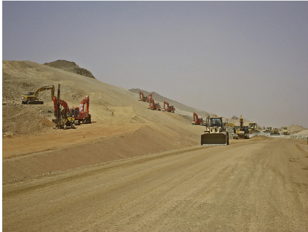
Fig. 4 Excavators working on a high-speed rail construction site in Saudi Arabia give the appearance of an army of ants eating the land. Photo: Courtesy of Vicente Mayordomo. INECO (February 2017).
