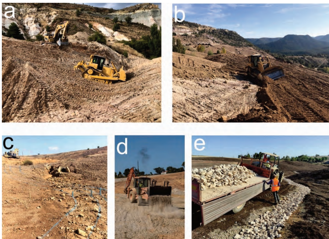
Figure 7 Images of the construction phases: (a) Bulldozer and excavator sculpting a valley in Peñalén (Spain); (b) Bulldozer spreading topsoil (carbonatic colluvium) and regrading a zig-zag valley in Peñalén; (c) Meandering channel staked out for building in Lousal (Portugal); (d) Backhoe excavator spreading limestone gravel (soil cover) at Lousal; (e) Building process of an open limestone meandering channel at Lousal
