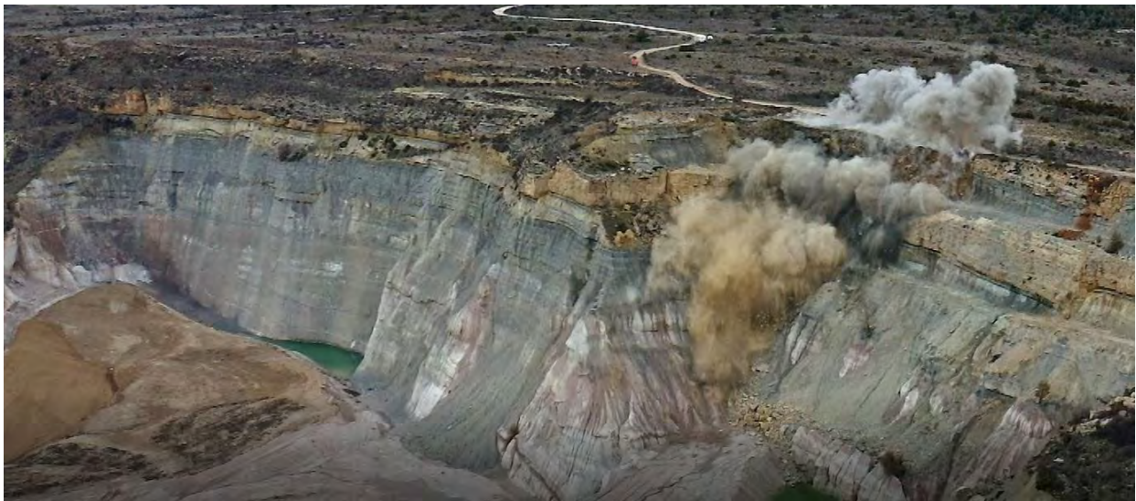
Figure 8 Blasting process at the higher positions of the Santa Engracia (Peñalén, Spain) residual highwall; first phase for replicating natural cliffs following the Talud Royal method (image by Miguel Ángel Langa)
