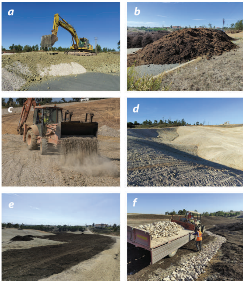
Figure 10. Execution of soil cover and AMD remediation actions: a) and b) materials used in the construction of the soil cover, limestone gravel and clays (a), and animal manure and topsoil (b); c) extension of the materials over the rehabilitation area with a backhoe; d) view of the intervention area after the extension of the soil horizon B; e) view of the first stages of the extension of the soil horizon A; f) lining of limestone blocks over the GeoFluv designed channels.
